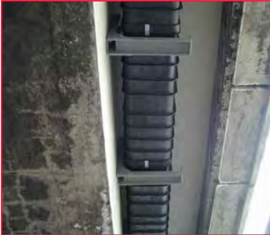
Example of a standard bridge crossing installation and bracket system.
